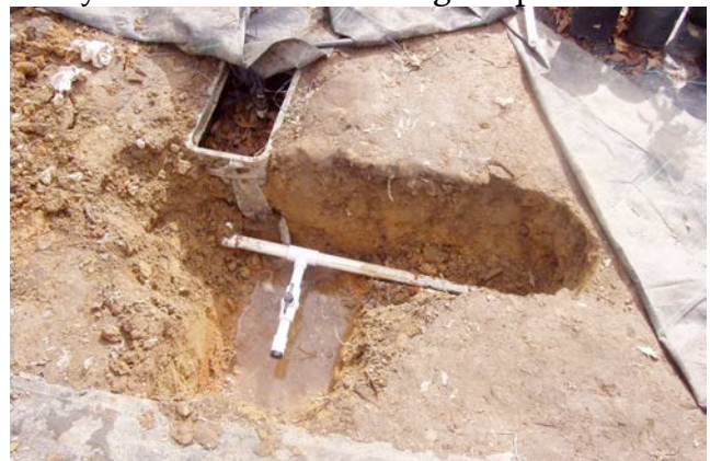
Detail of the automatic drain valve recently installed at the nursery. Photo by Don Crowder, 2012.
